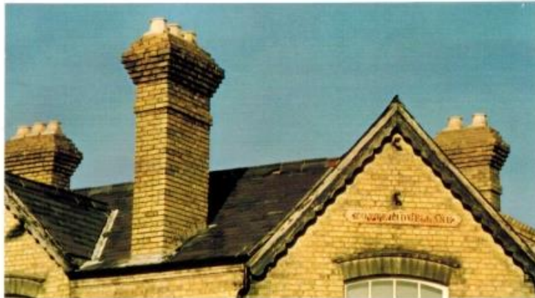
Gone forever. The lovely roof over Harper's in November 2000, just before demolition.
