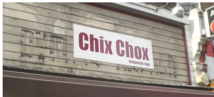
In January 2012 the fascia of number 793 High Road, North Finchley was removed, to reveal that of Pymmes Kitchen which was there in 1975
